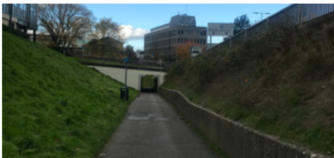
Figure 7.4: Subway on approach to the town centre from the east with Easthampstead House in the background
